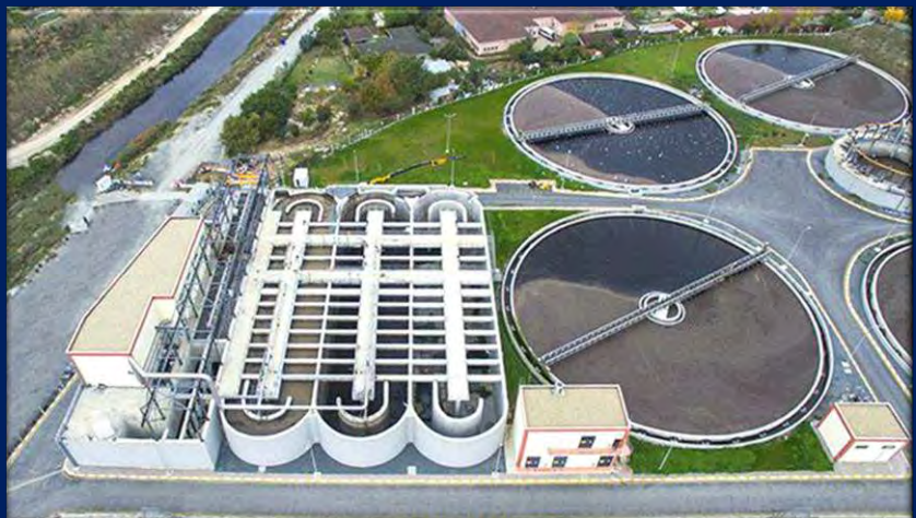
Atakoy Wastewater Reuse Plant – Istanbul, Türkiye.
