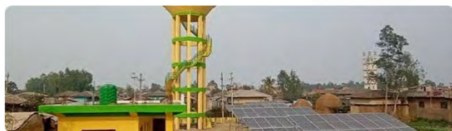
Solar-powered lift station feeding an elevated storage tower
