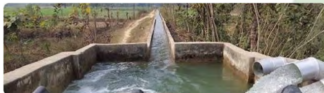
Lifted water discharging into a field irrigation canal
