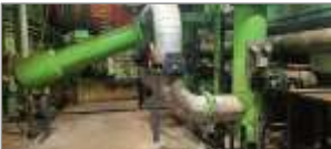
Protected pump-house piping & valves Source-level treatment keeps downstream pumps, valves and gauges silt-free — extending the life of the whole network.
