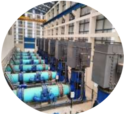
Pump House Automation
